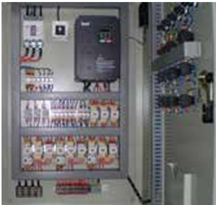
Electric control panel – Contactors, overload relays, inverters and main isolator in an IP-rated enclosure.
